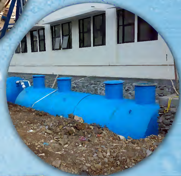
FRP TANK - HORIZONTAL TYPE ON-SITE
